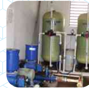
Sewage Treatment Plant (STP)
