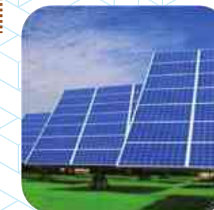
Solar Plant & 24x7 DG Power Backup in Common Area
