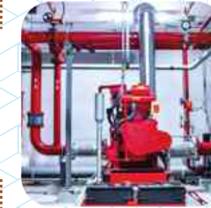
Fire Fighting System
